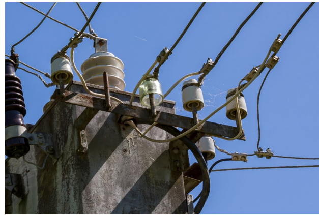
Electrical grid © AdobeStock / Valeriya
