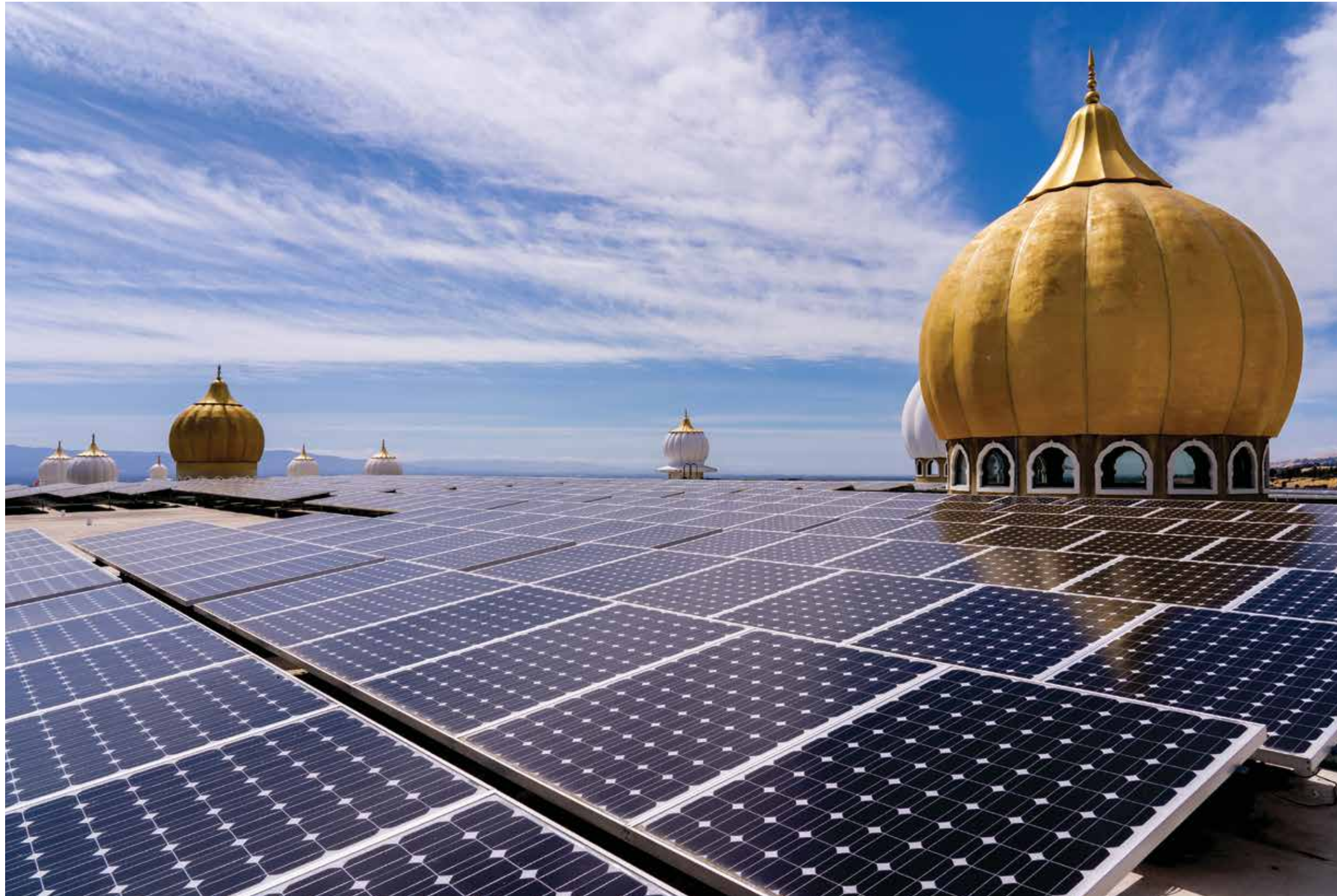
San Jose Gurdwara Solar Panels. Photo by Meeka Studio.
