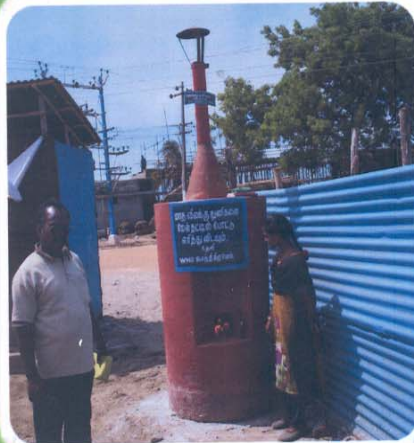
masonry Incenerator disposal of Sanitary Napkins constructed at Nagapattinam Temporary shelters near the women toilets
