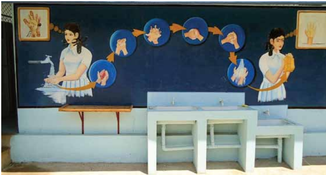
Child Friendly School toilet in Vellaveli, Batticaloa, Sri Lanka, with hygiene promotion message
