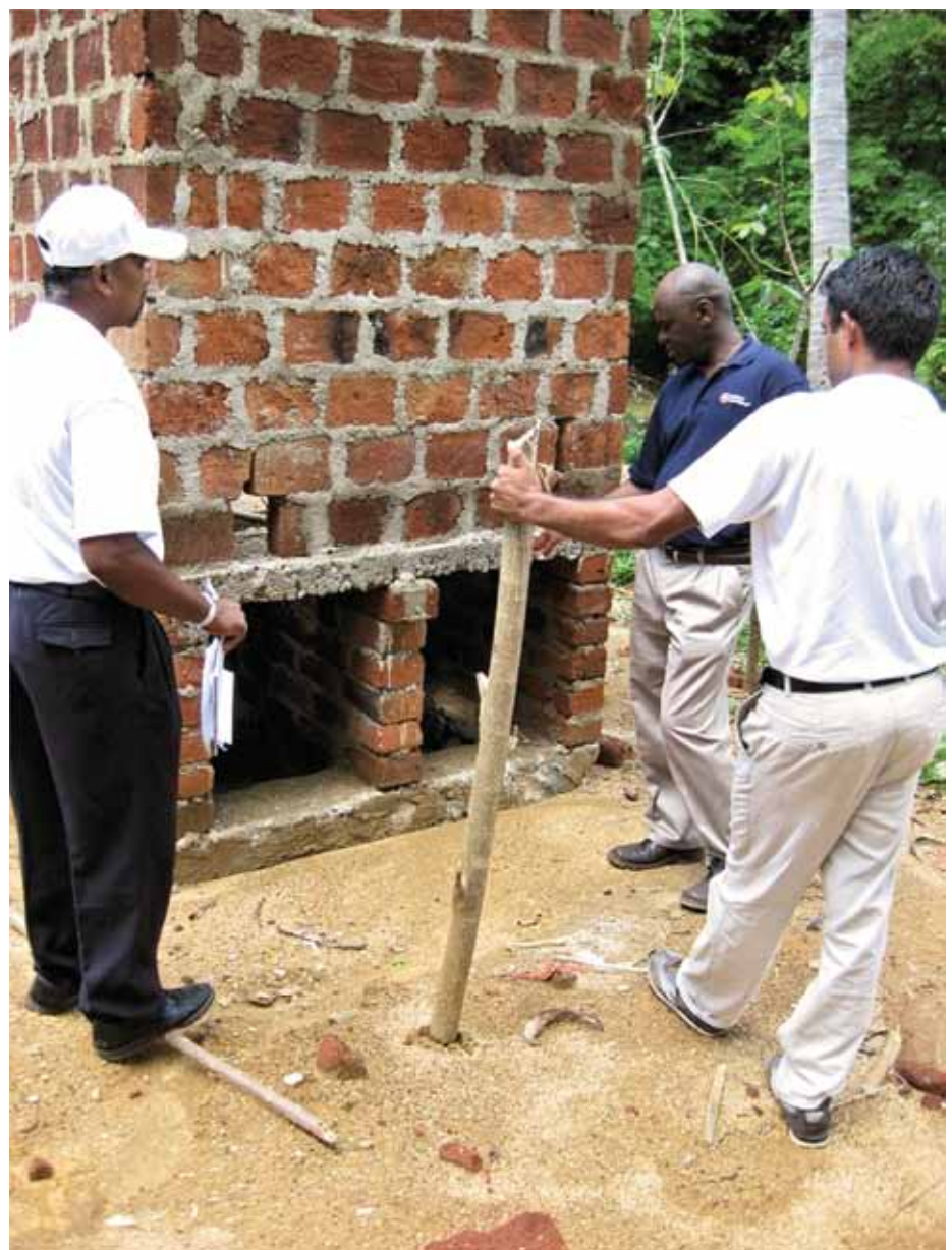
Dry double pit compost latrine under construction in Sri Lanka, the double chambers under the latrine are clearly visible
