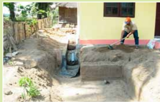
Construction of a wetland and leach field where the pre-treated effluents from the Biofil tank are further filtered and finally released into the ground, Indonesia
