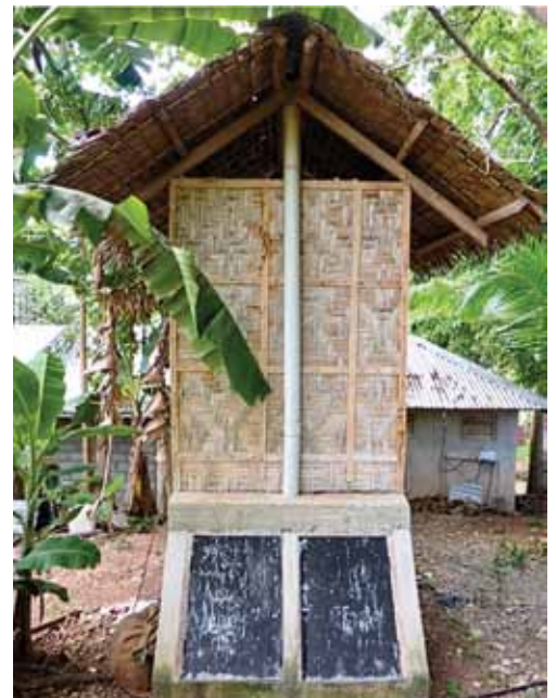
Double-chamber UDDT using local materials, Mindanao, Philippines (source: Robert Gensch 2009)
