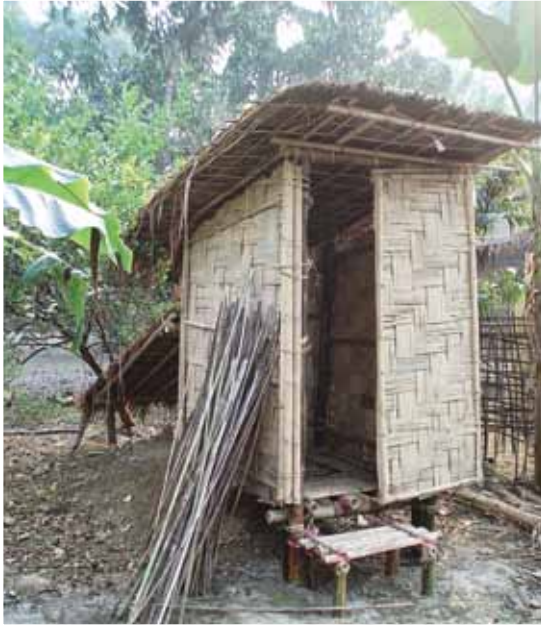
Completed latrine in Myanmar with off-set pit. Annex 1 shows the drawing and Bill of Quantities (BoQ) for such latrine with galvanised iron sheet roofing.
