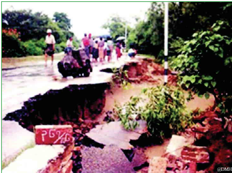
Damaged Yangon-Mandalay highway due to flood
