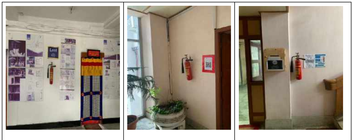
Figure 7: Fire extinguishers in the Ministry
