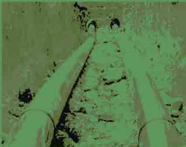
13. Water supply through pipeline
