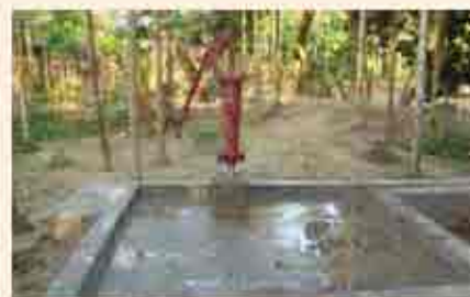
Platform is in good condition: drainage system is good, surrounding is neat and clean that means no waste and dirty water exist
