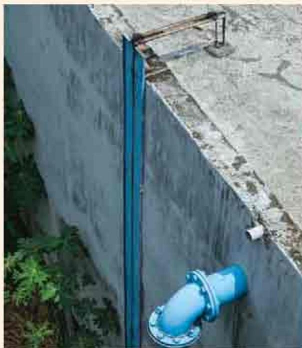
8. Water storage In ground reservoir
