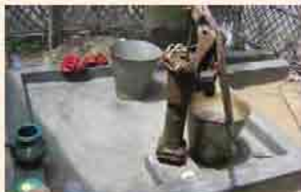
No lid on the top of the pump
