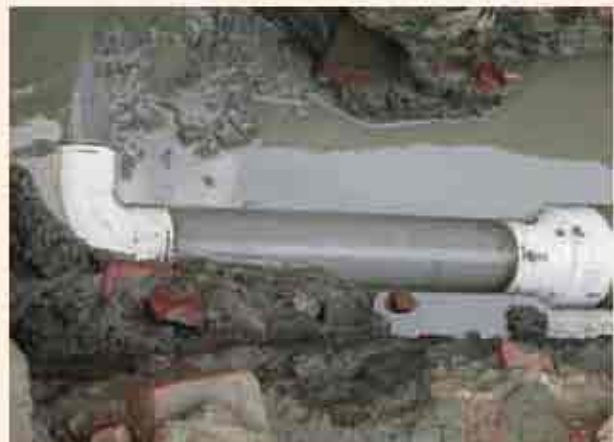
13. Water supply through pipeline
