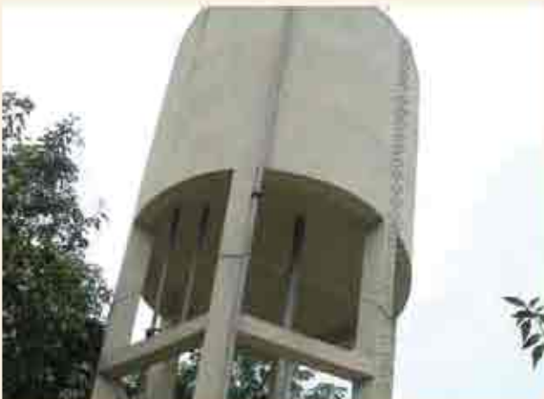
12. Water storage in overhead tank
