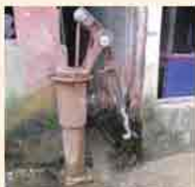
No platform or platform is damaged. Surrounding area of the platform is unclean with waste and dirty water around
