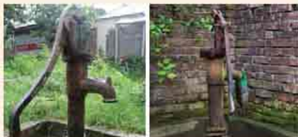
No sanitary seal, cloth/bottle is fastened at the mouth of pump
