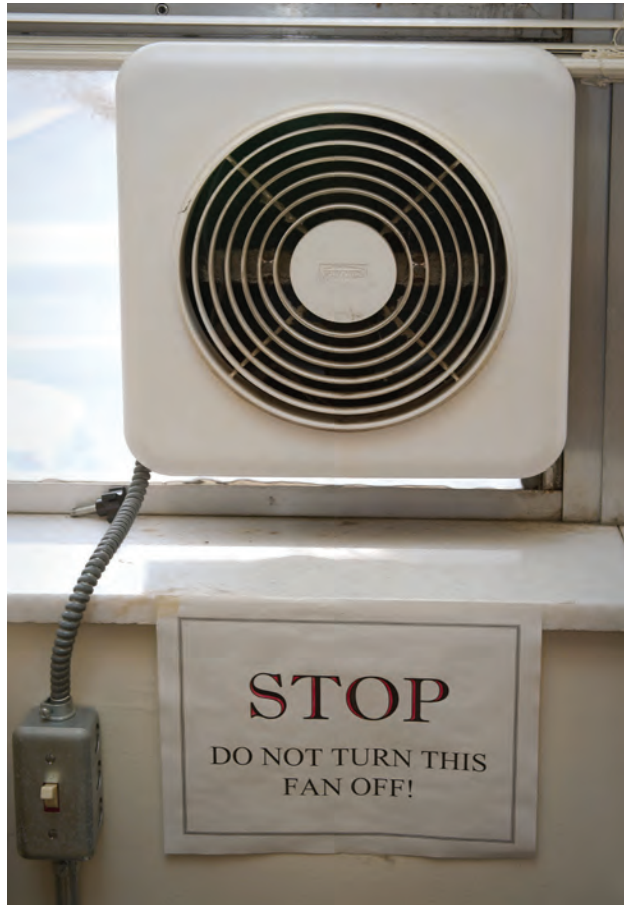
Figure 7.1 Exhaust Fan Used for Distributing Air
